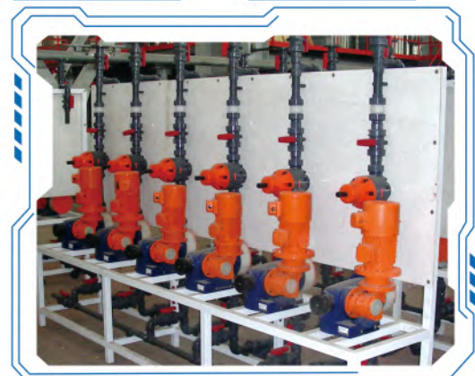
Dosing pump machine
